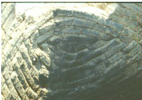
Fig. 9. An exacting brick pattern was required to reproduce the traditional ovoid shape of the dome.
